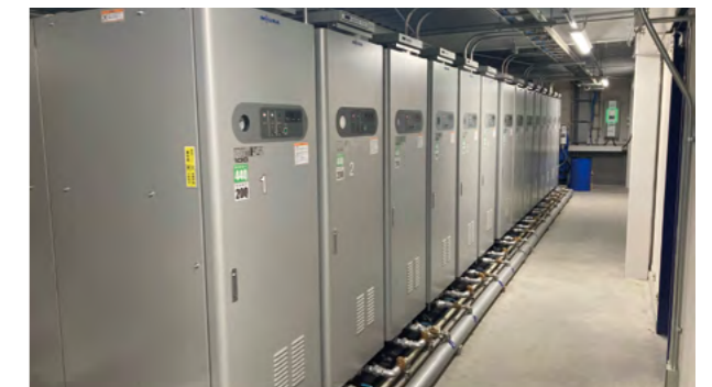
Newly installed electric boilers used in painting facilities
